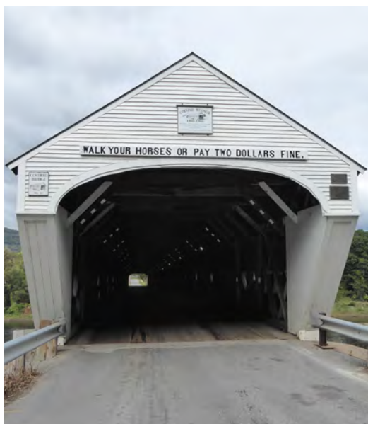
The Cornish-Windsor Bridge, crosses the Connecticut River between Cornish, NH, and Windsor, VT
