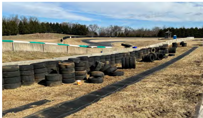
Conveyor Belt Tire Wall under construction on the Shenandoah Circuit. The tires are stacked, connected together, then sandwiched between the back wall and a conveyor-belt strip on the track side
